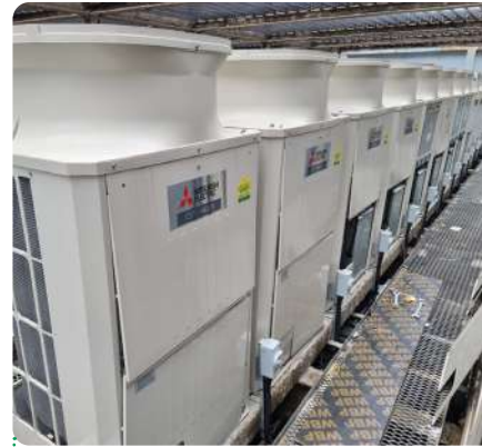
VRF condensing units at lyf Bugis Singapore where the efficiency and cooling capacity were measured.
